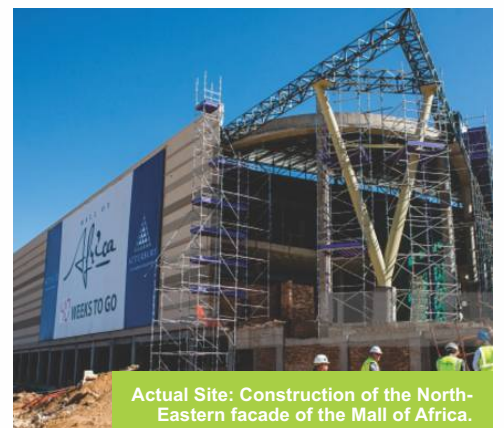
Actual Site: Aerial view illustrating the progress of construction on the roof of Mall of Africa.
